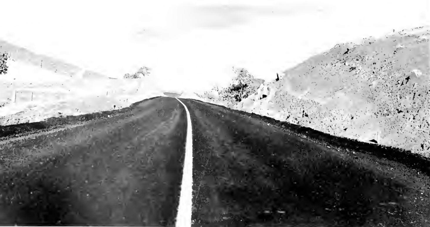
Section of new, wide two-lane highway with bituminous mix surfacing recently completed on Cholame lateral through Cottonwood Pass
